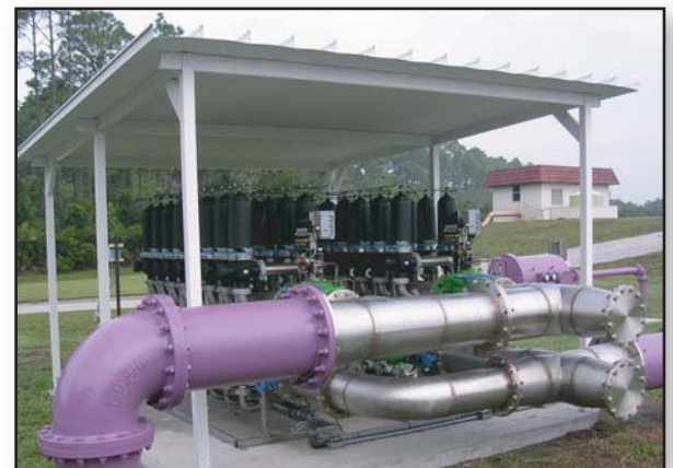
Dunes Utilities – Reclaimed Water Filter Station. Filtering Reclaimed Water used for Irrigation.
